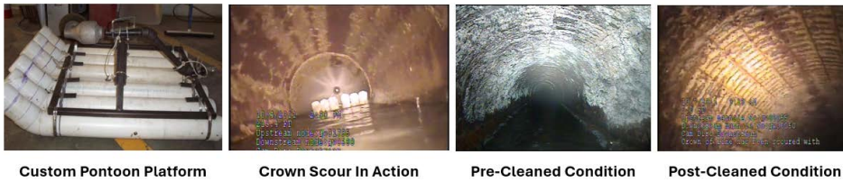
Fig. 5. Cleaning Pontoon Fabricated with Controllable Jet Nozzles Tethered to Remote CCTV System Inside NPSSI
