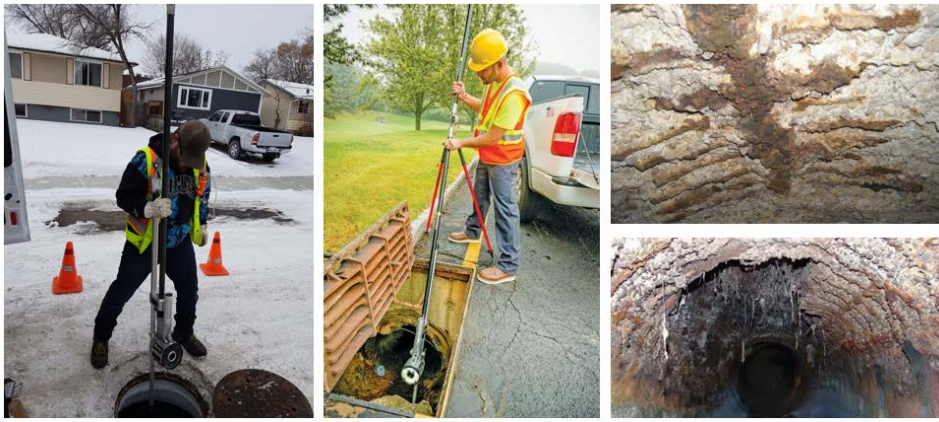
Fig. 3. The Envirosight Quickview® System Used for Initial Top-Side Inspection of NSPPI
