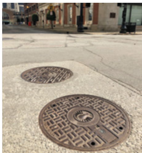
Explosion Mitigation assembly Louisville, Kentucky.
