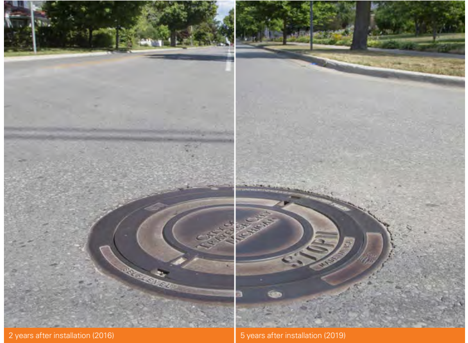
SELFLEVEL access assembly installed in Traverse City, Michigan.
