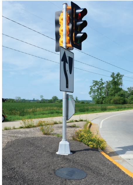
DUROCOM handhole installed near traffic lights.
