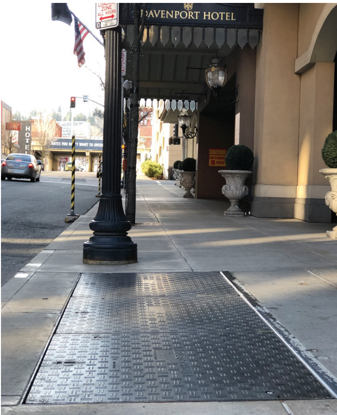
These ergonomic composite covers were retrofitted in steel frames in downtown Spokane, Washington, replacing old steel grating which was allowing salt and other road debris to fall directly on top of the power transformer below.
