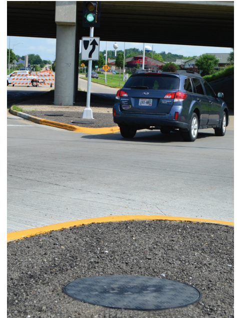
DUROCOM handhole assemblies installed.
