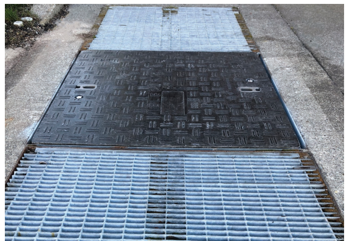
This composite panel replaced a broken section of grating located directly over the vault's access ladder. The retrofit installation was the perfect solution—leaving the remaining grating to provide ample ventilation for the power structure below.
