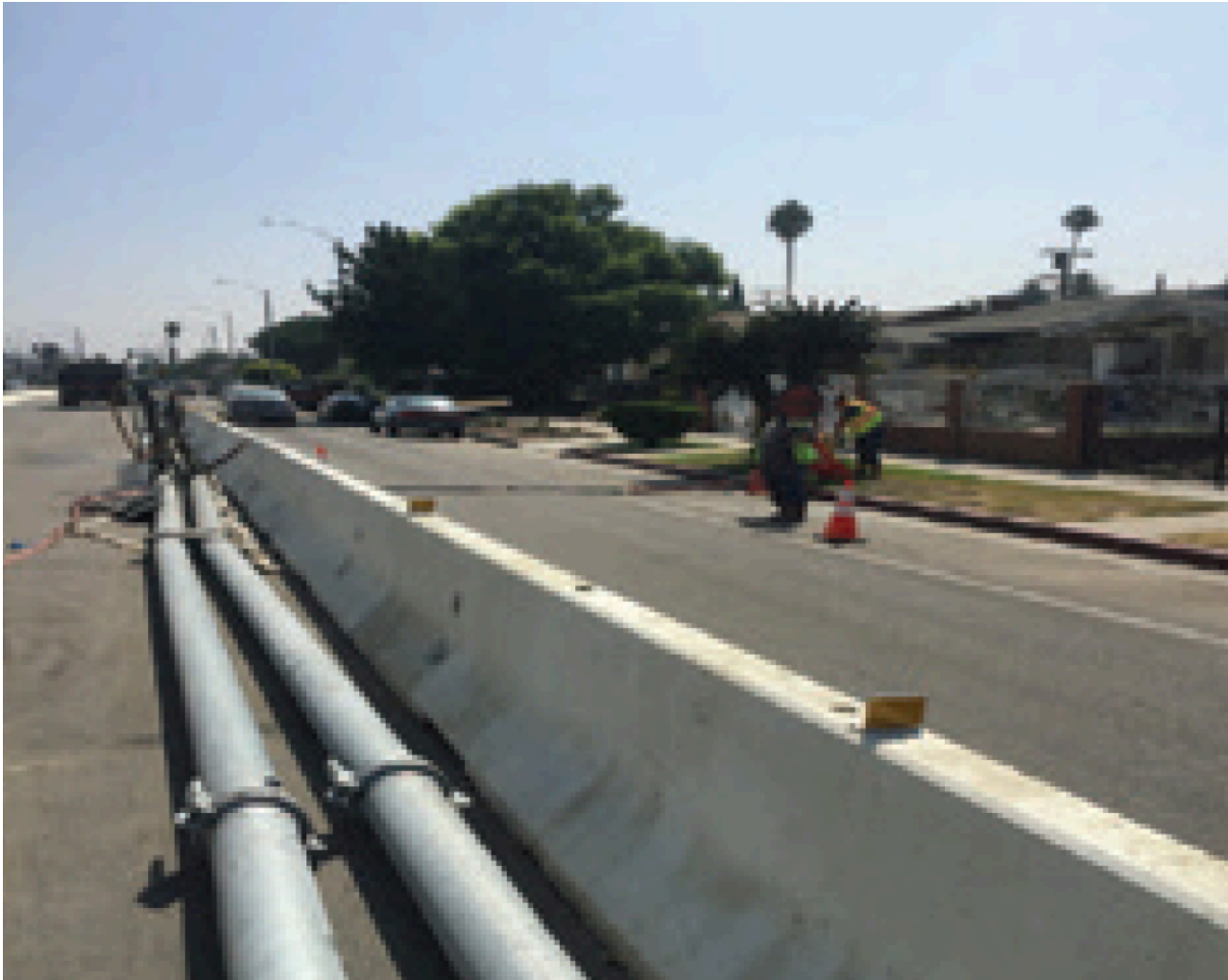
A bypass system was used along Rodeo Road during the lining of a brick sewer underneath.
