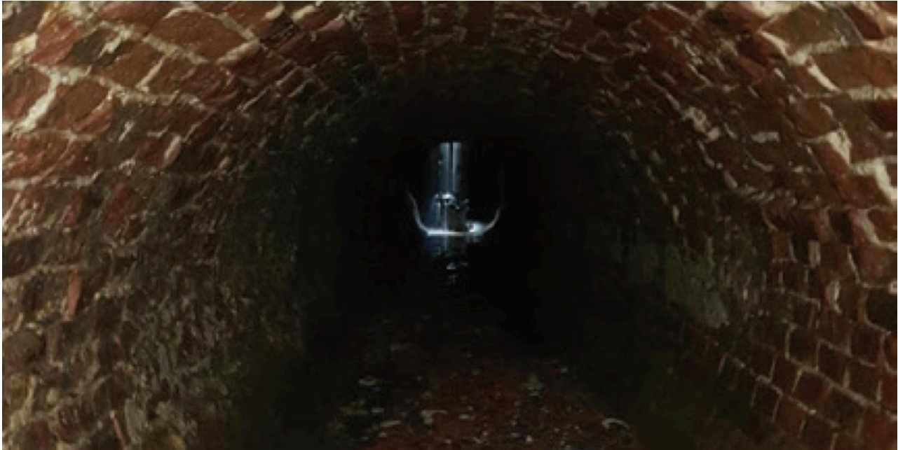
Initial brick structure with debris and missing mortar.
