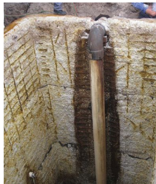
Biogenic corrosion of Portland Cement
