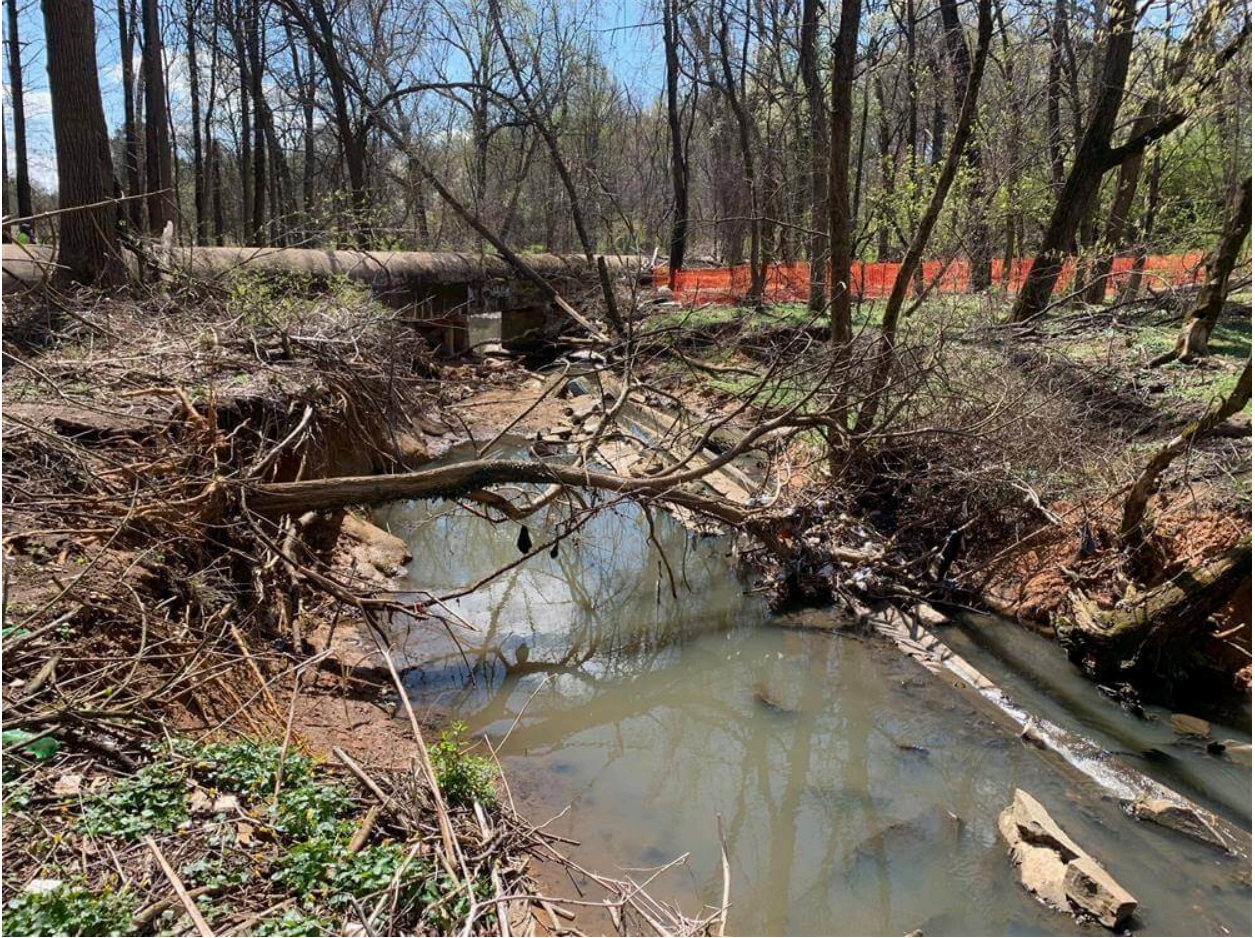
The aerial sewer crossing was significantly impacted by surge flow and required an emergency design-build repair
