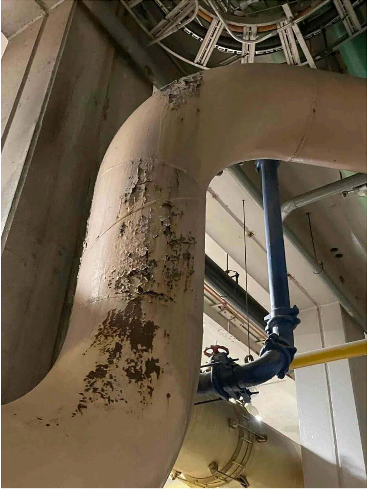
Return Activated Sludge (RAS) piping system before repairs
