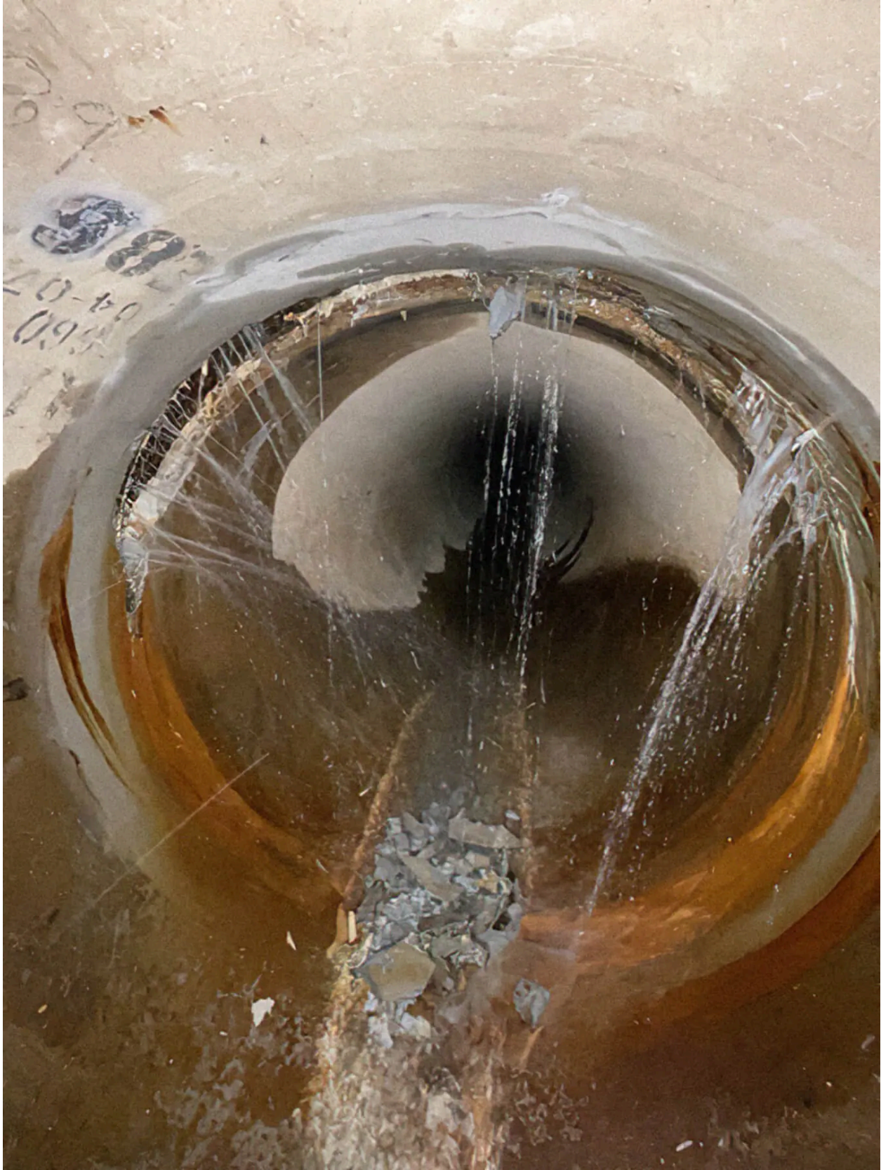
Wire breaks in Prestressed Concrete Cylinder Pipe (PCCP)
