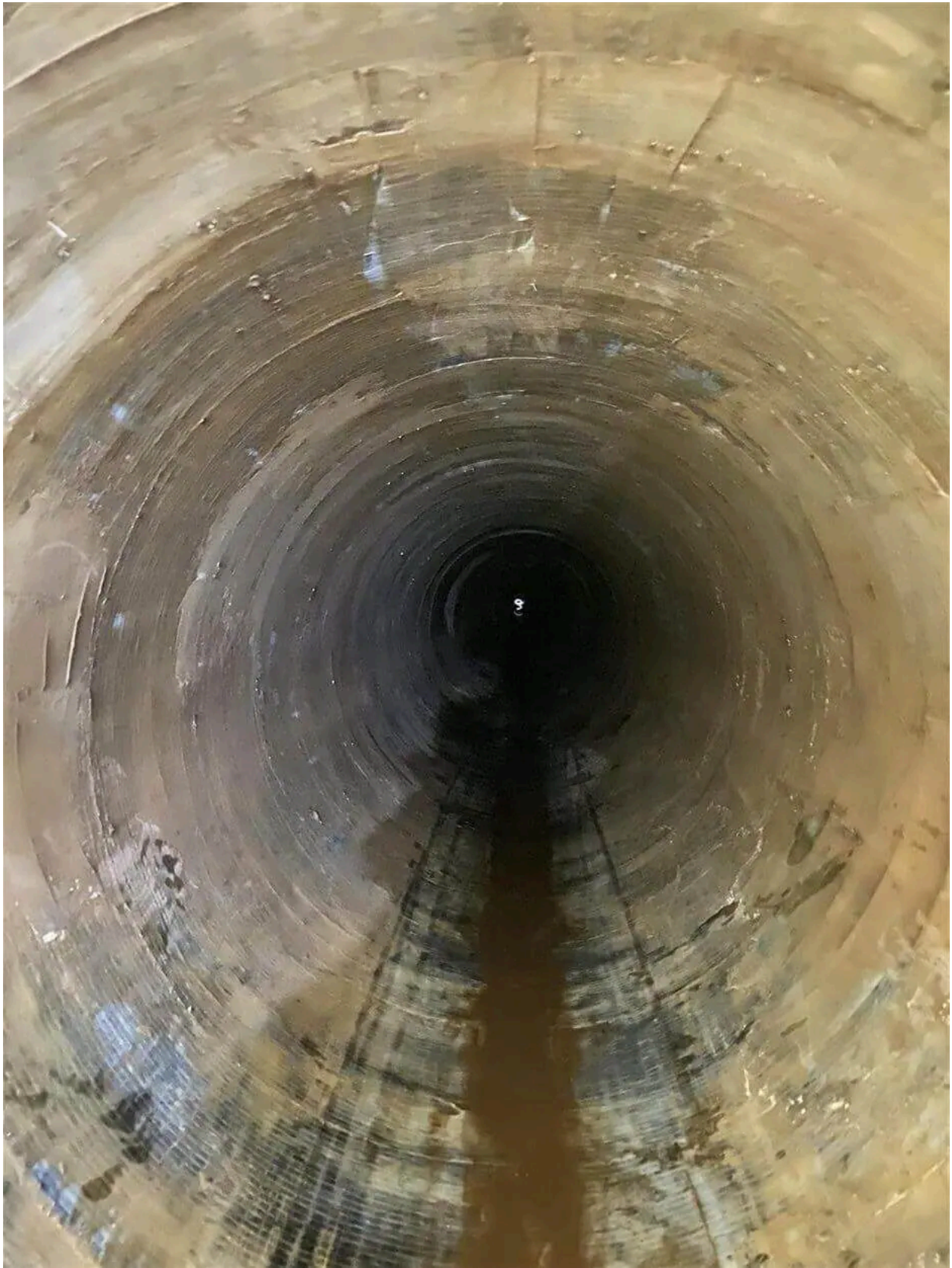
Pipe section before repairs.
