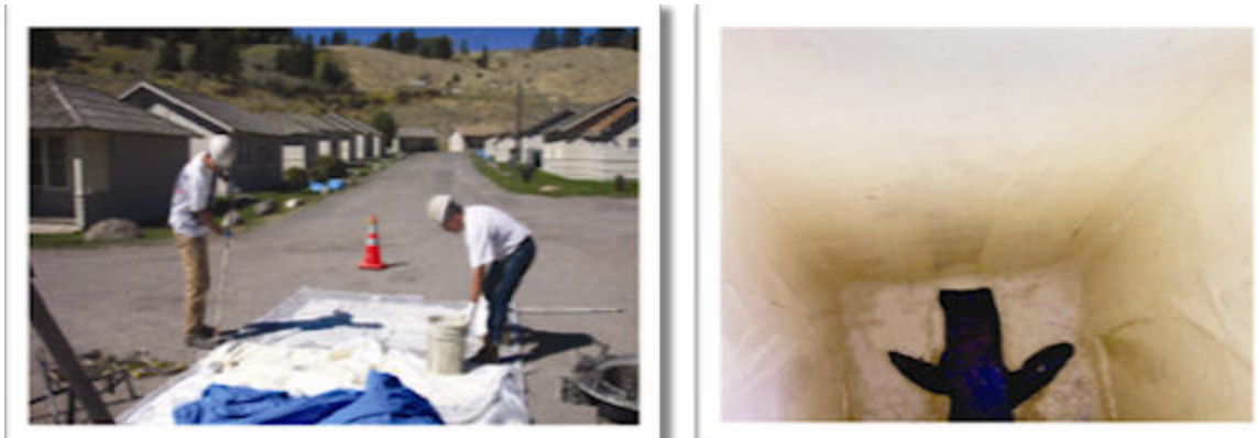
Upper Left: Liner is being saturated at the jobsite with 2-part epoxy resin.
