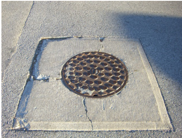
Cracking due to
