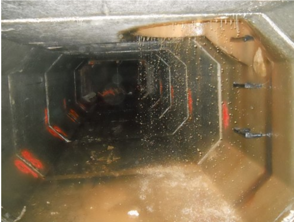
Leaking manholes add to the groundwater infiltration
