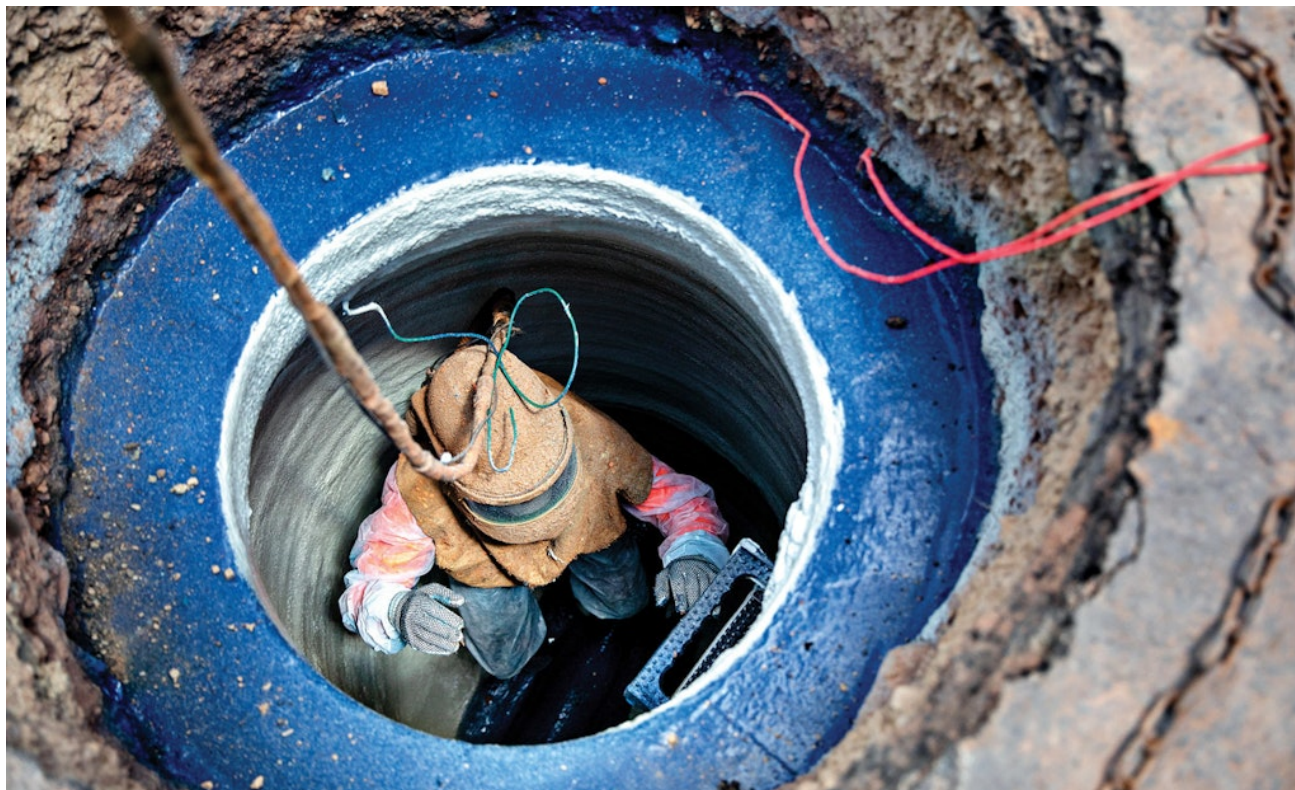
Technician Austin Huggins installs a liner inside a new manhole in Park City.
