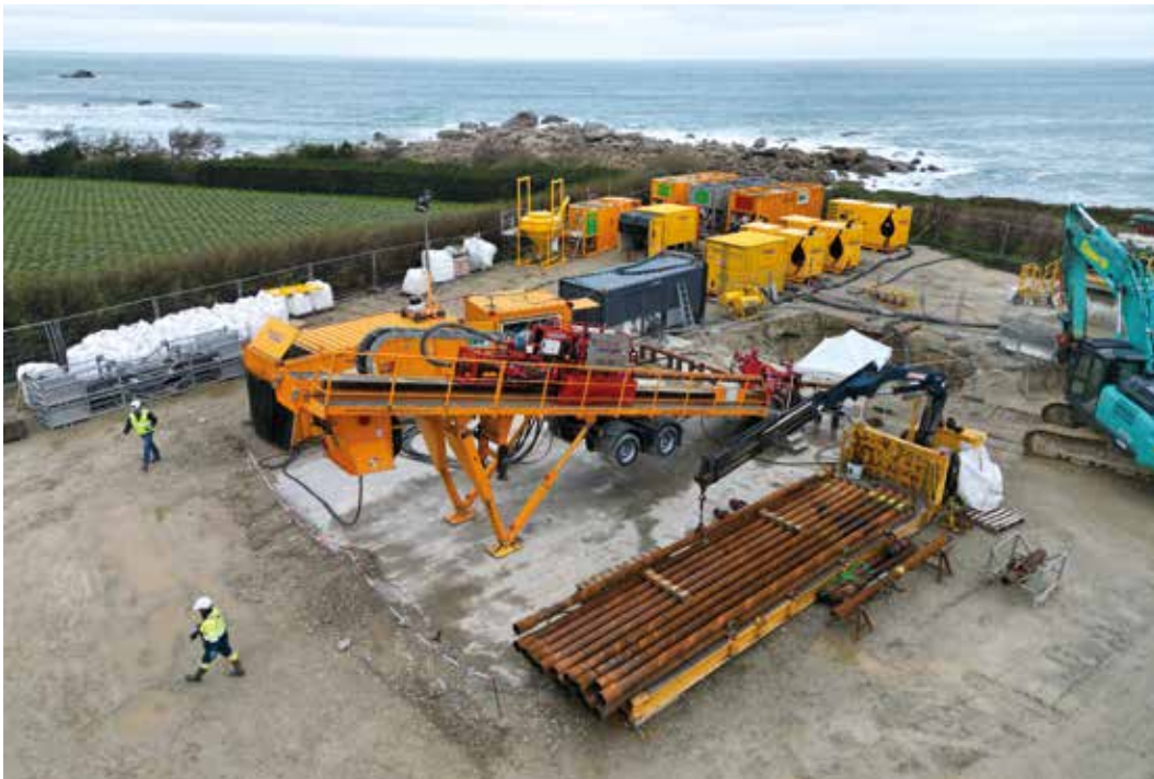
On the jobsite: HK250T Trailer Rig in operation, for cable landfalls on the coast of Brittany, France
